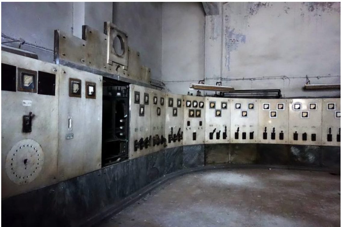
The control panel of the turbine house. March 17, 2017 Photo by N. Dushkina
