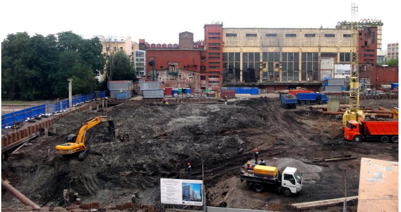
Excavation of the foundation pit for the Mendelsohn Residential Complex. Friday, July 22, 2016 Photo by S. Gorbatenko
